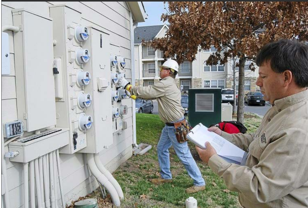
AEP-PSO field revenue specialist Brian Gross changes out old meters for smart meters at a University of Tulsa campus apartment complex while field services supervisor Mike Ruley notes final readings on old meters. Courtesy
