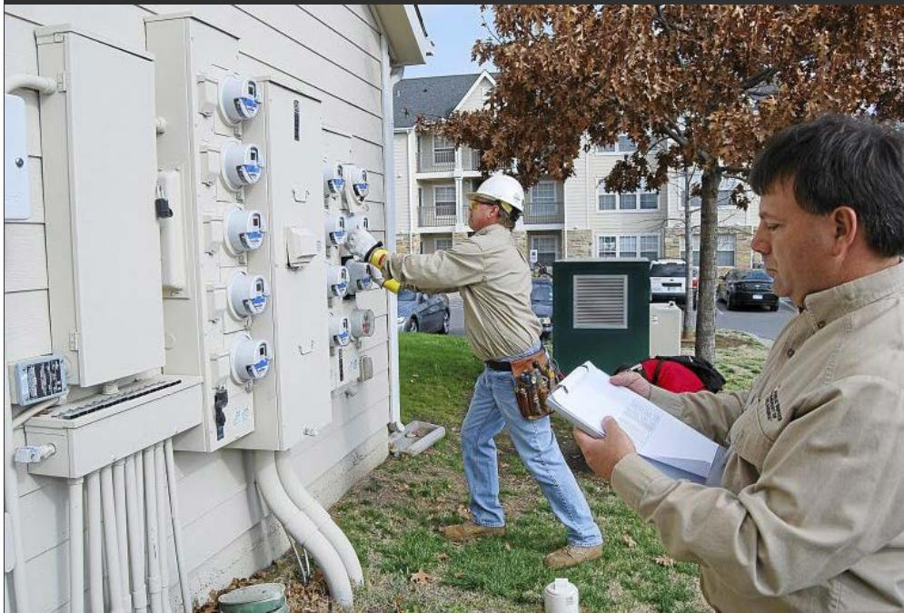
AEP-PSO field revenue specialist Brian Gross changes out old meters for smart meters at a University of Tulsa campus apartment complex while field services supervisor Mike Ruley notes final readings on old meters. Courtesy
